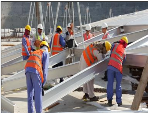
NWC's TGSW, Salboukh site, Riyadh, Saudi Arabia (ID 110m x 12 Tanks, 2017)
